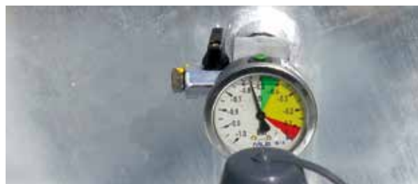
Vacuum leakage monitoring
